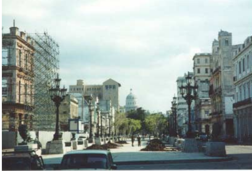
The Prada, viewed while looking towards the Capitolio in Havana. Scaffolding can be seen showing the restoration underway in this historic area of the city.
